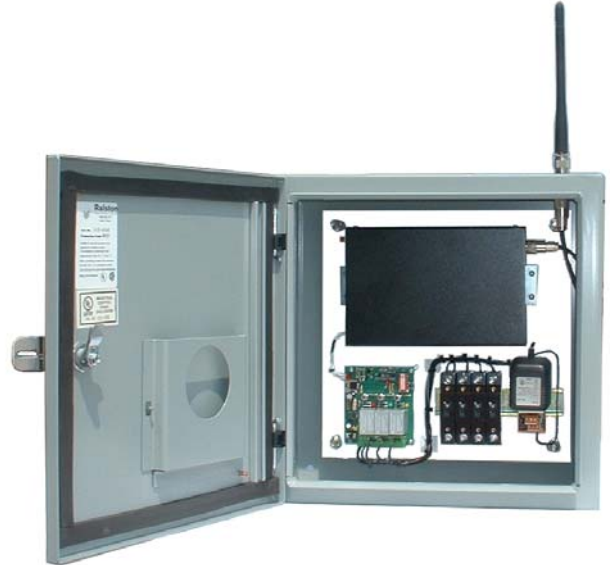
Radio control installed in NEMA 4 box.
